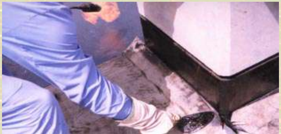
Base Flashing Needs Special Handling.
